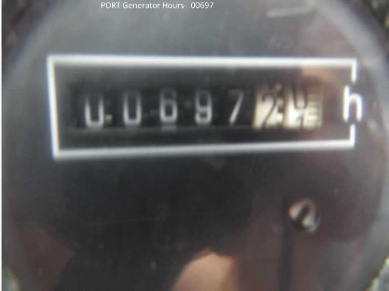
PORT Generator Hours- 00697
